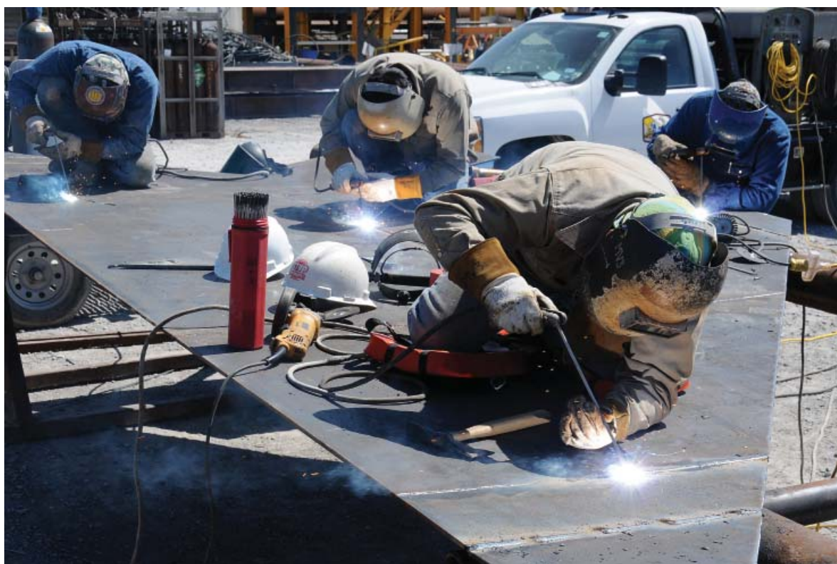
PORT FOURCHON, La. – A team of welders fabricates a portion of the subsea oil recovery system chamber. The chamber will be one of the largest ever built and will be used in an attempt to contain the subsea flow of oil. Photo courtesy of U.S. Coast Guard
